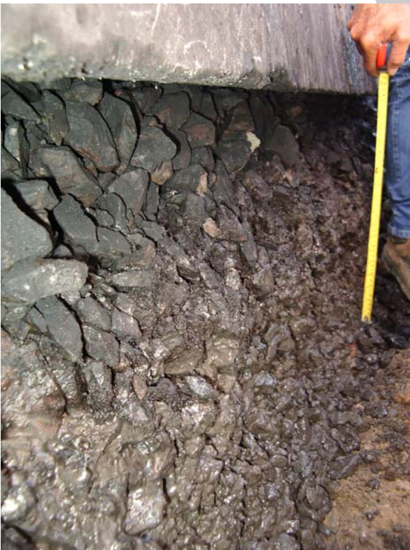
Figure 2: Ballast highly fouled mixture of degraded ballast and some coal fines (formation intact)
