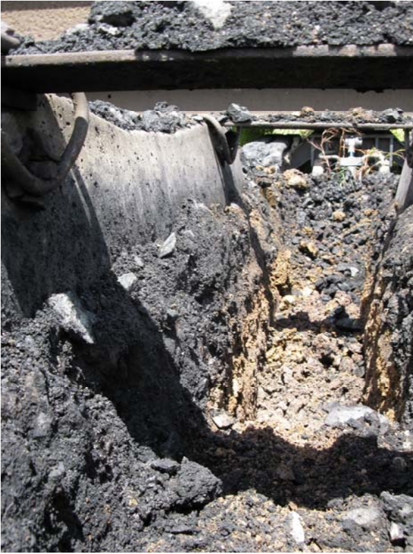
Figure 1: Ballast highly fouled with coal
